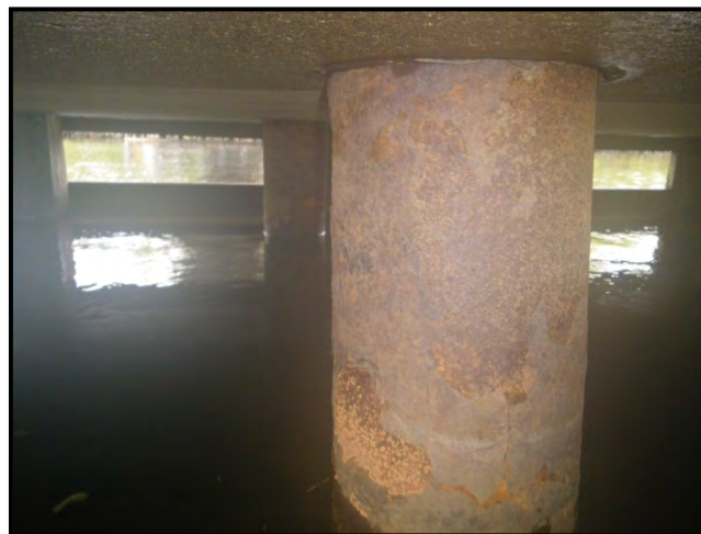
Figure 2-22 Typical Steel Pile with Moderate Rusting
