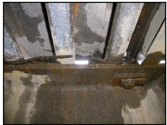
Figure 2-14 Loose Deck Connection, Broken Neoprene
