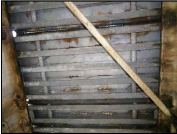
Figure 2-13 Typical Deck Panel Condition
