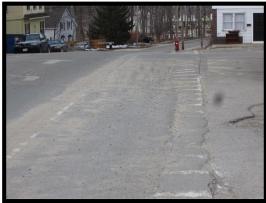
PHOTO16: GAP IN SIDEWALK ALONG GROTON ST
