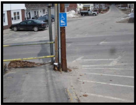
PHOTO 14: ACCESSIBLE RAMP IN FRONT OF SPA CAFÉ IN POOR CONDITION
