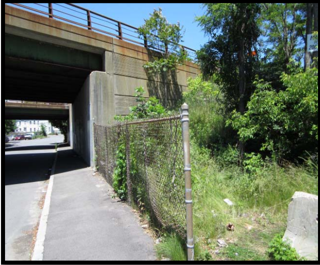
Photo 5; Break in the chain link fence on Lincoln St.
