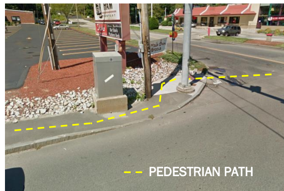
The placement of the sign post, utility pole and utility box on the corner of Silver Drive and Daniel Webster Highway obstructs pedestrian flow on the sidewalk.
